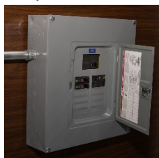
Surface Mounted Panelboard
