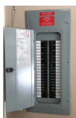
Flush Mounted Panelboard
