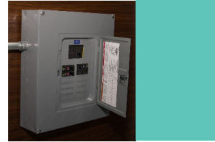
Surface Mounted Panelboard
